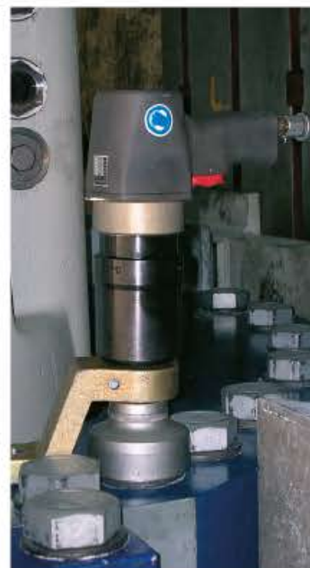
alkitronic® CLD torque multipliers in use (figures on the right). Screw connections at a bolt circle and a diesel unit for large construction machines
